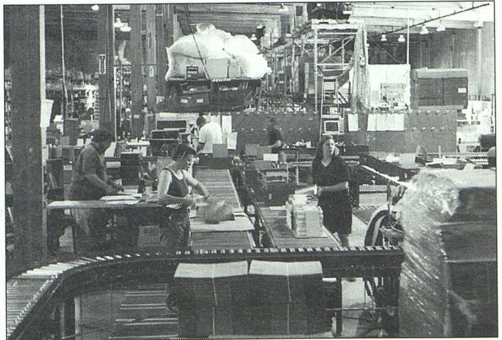
1996: A crew works to install the new packing/shipping line in the Oakland warehouse.
