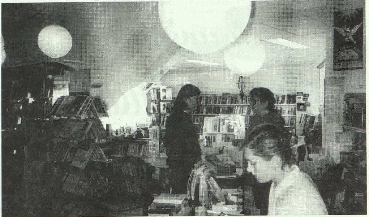
Removing the wall between two shops doubled the size of the Sydney shop.
