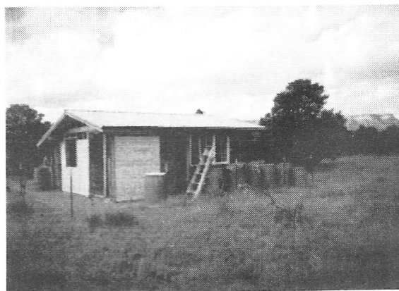
Rebecca's house: This house has an interior dimension of 14' X 14'. 2½ walls are straw bale and the others are a combination of doors, windows and paneling.
