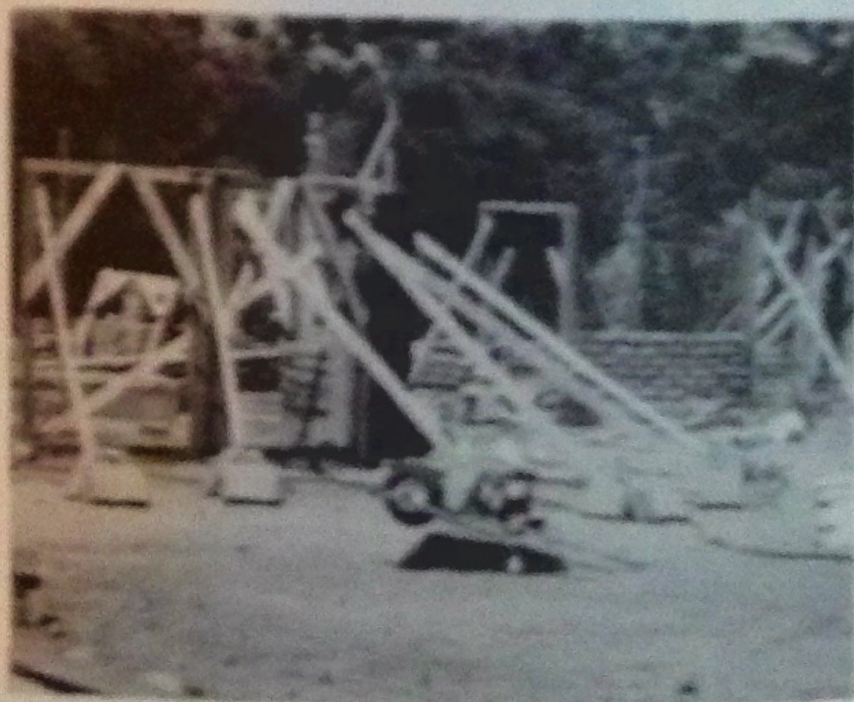
Squared and plumbed door and window frames. Vee on outside where frames join. Wood plate on top helps secure frames together. Braces are tagged with flagging tape to save Dyke heads. We're starting to lay the adobe blocks between frames.
