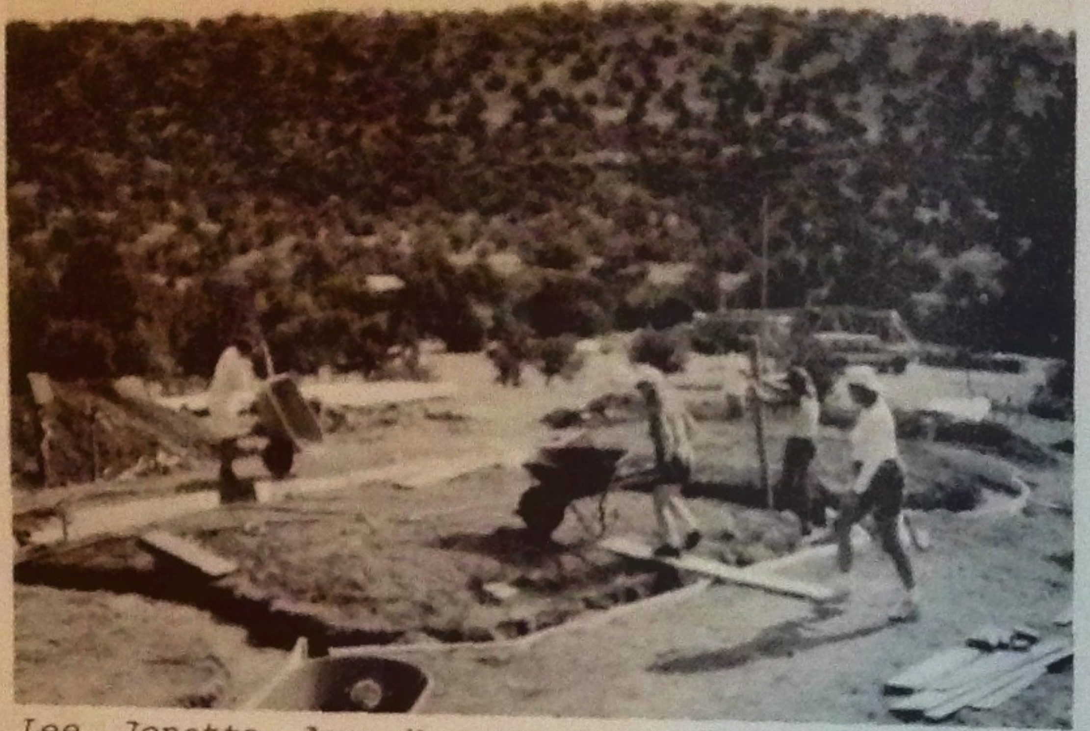
Lee, Jonetta, Ame, Karen and JC filling and tamping the sand/gravel floating footing. White line on outside of footing trench is underground insulation.
