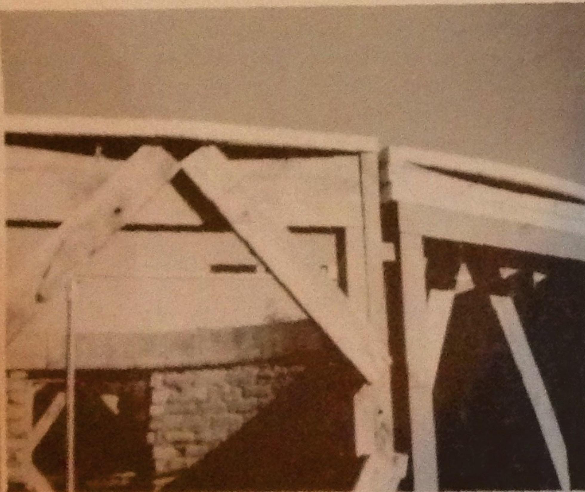
Arcs made from 2x6's are secured to the top of the frames to shape the round of the bond beam. Extra boards are placed on top of shorter frames (right) to flush them to wall height.
