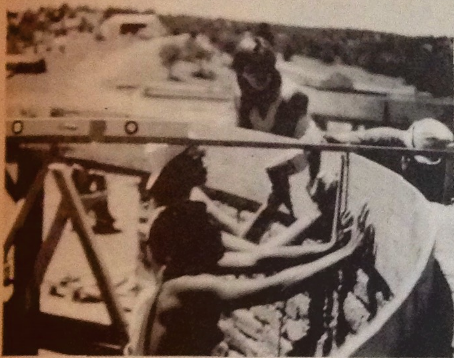
Miguela, JC, Karen and Ame using center pole to level bond beam forms. Form is screwed into gringo blocks in the top row of adobe.
