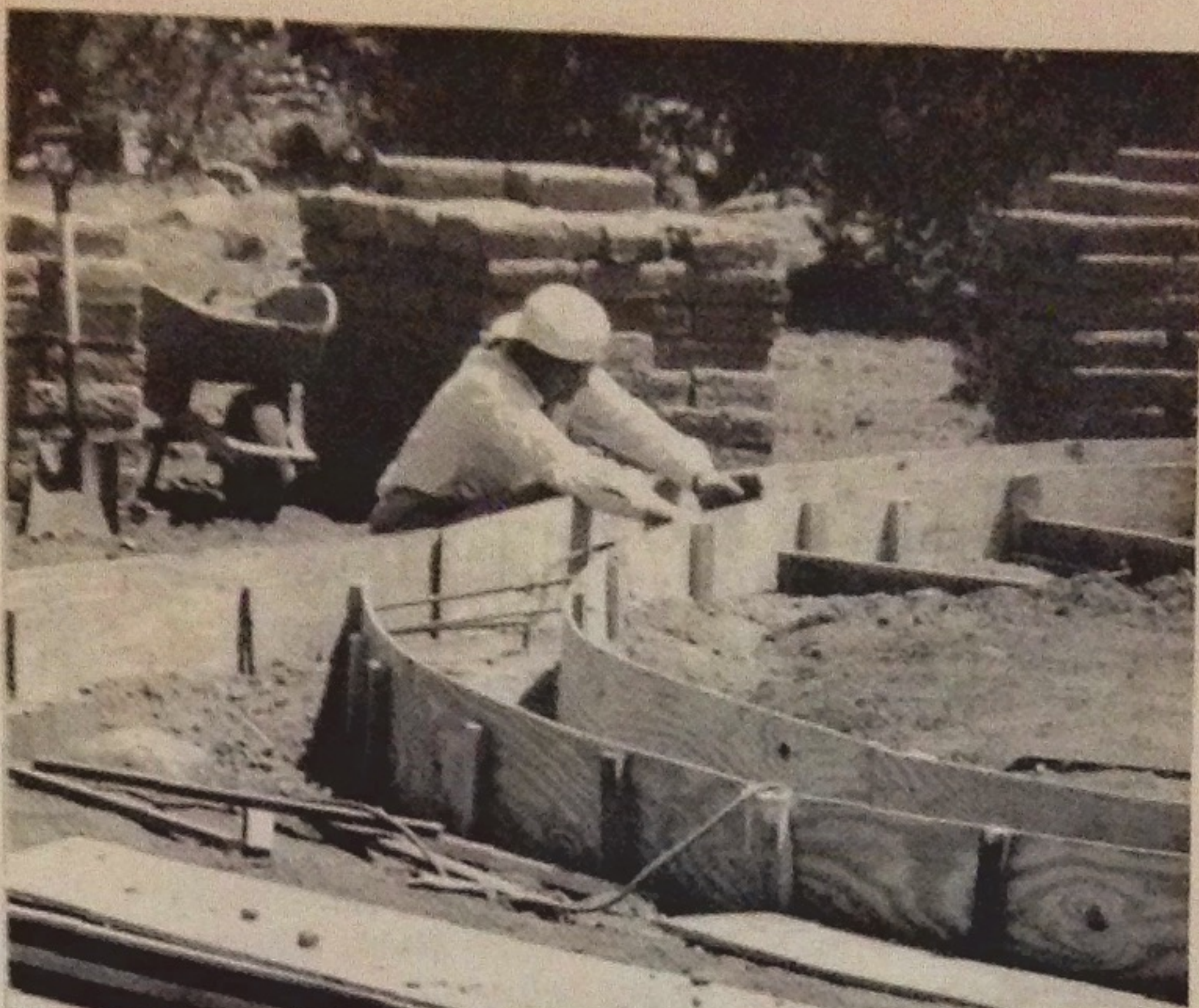
JC ties rebar to wire twists that hold plywood stem forms 14" apart, the width of the adobe wall. Concrete stem is at least 8" high.
