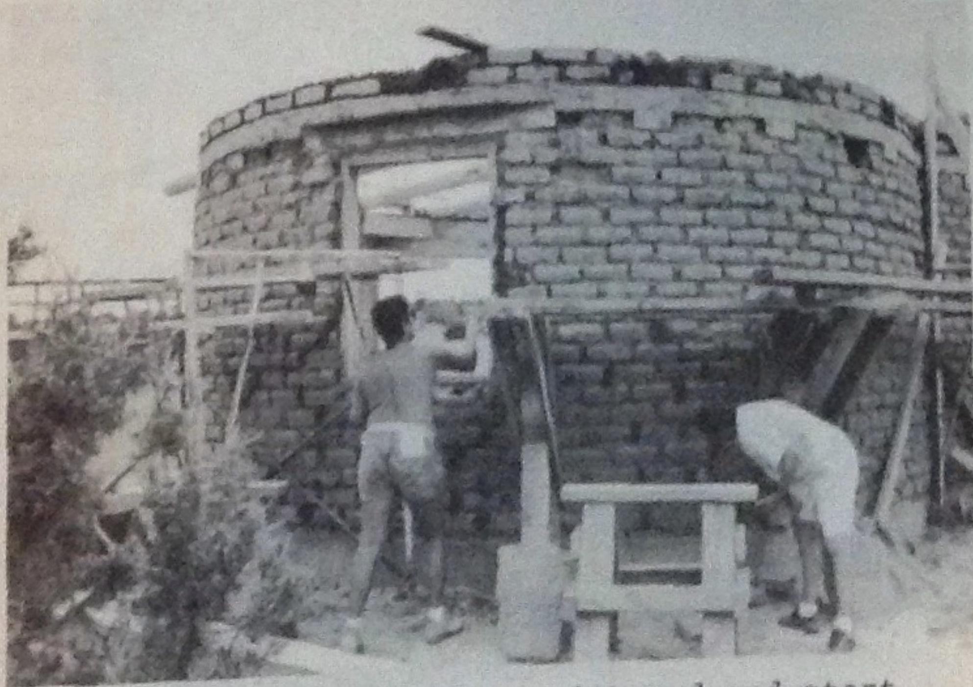
Lua and Lee fill holes with mud and start rounding out wall around window. Lintel extends over window frame 1' on each side. Concrete bond beam and the gringo blocks that held the bond beam form show well.
